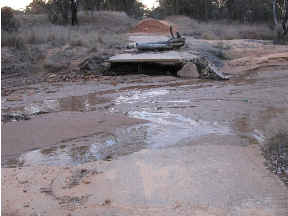
Flood Damage to Concrete Causeway on Box Ridge Road at Yallagal Creek. Significant planning was undertaken to replace the damaged section of road with a box culvert drainage structure.
