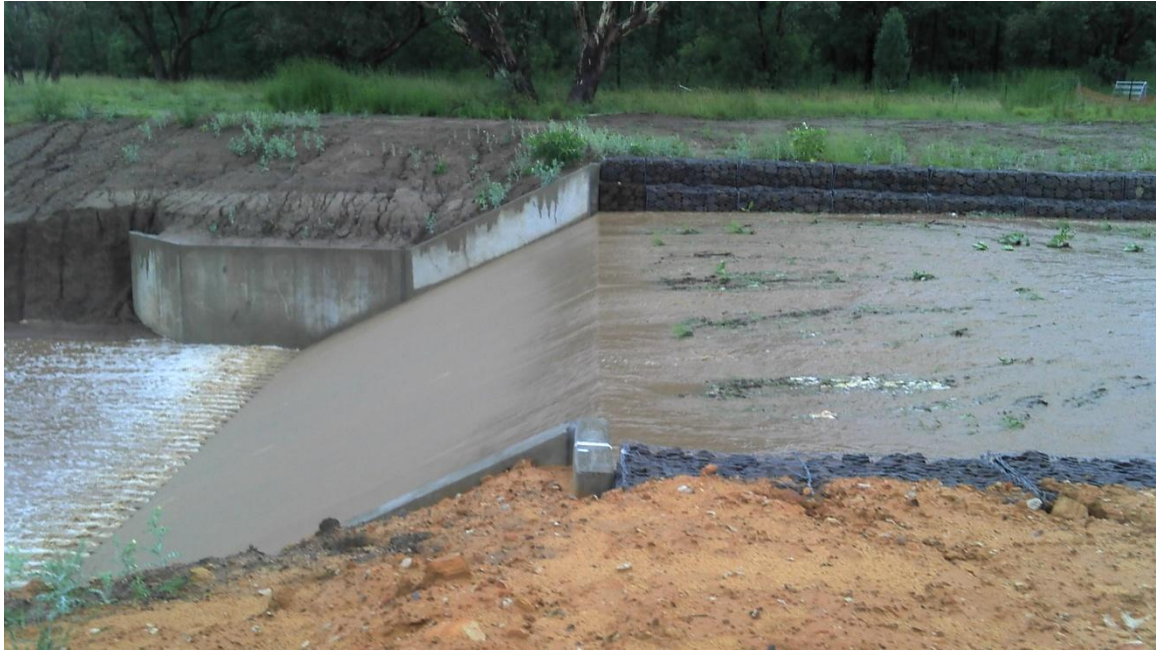
Stabilisation of Teridgerie Creek downstream of the causeway on Bugaldie Goorianawa Road involved construction of a large concrete flume and rock lined channel.
